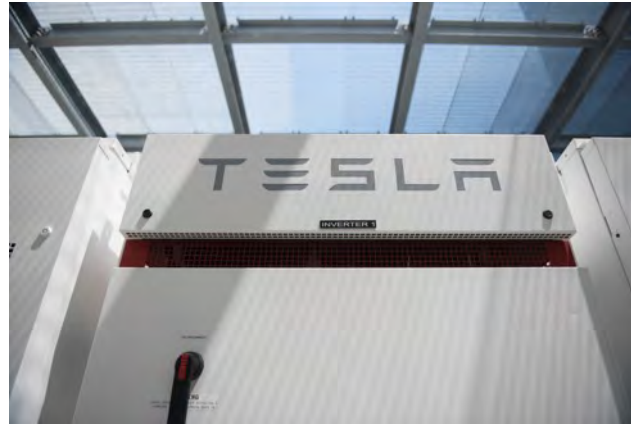
Battery Energy Storage
